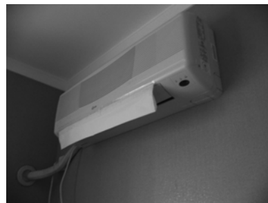
Fig. 15. Housing not designed for installing for split-unit air-conditioners as shown by the exposed duct.
