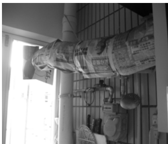
Fig. 14. Housing not designed for installing kitchen cooking hoods.
